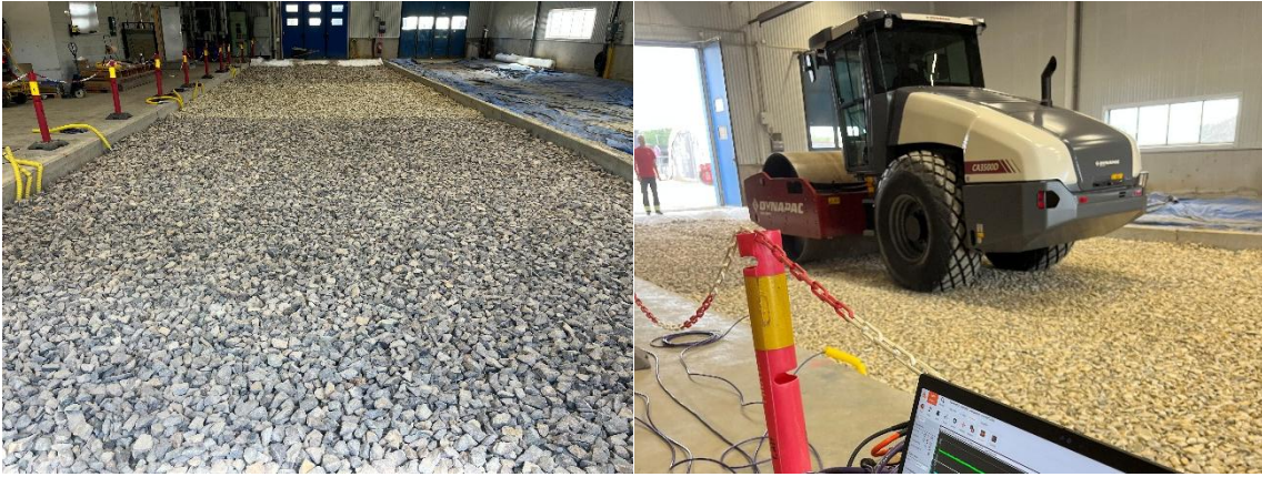
Figure 8. Left: channel filled with material M1-M3 before static compaction. Right: During static roller compaction.
